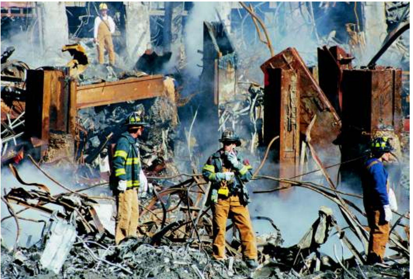
Figure 3-5 The core column in the center appears cut by a torch. The workers cut the steel so quickly that it is difficult to determine which damage was from them.
